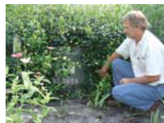
Assistant Operations Manager Glenn Parks inspects an overgrown transformer.
