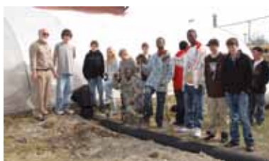
Stephen Karl and his students dig a trench that will hold the piping used to transfer warm greenhouse air to a nearby classroom.
