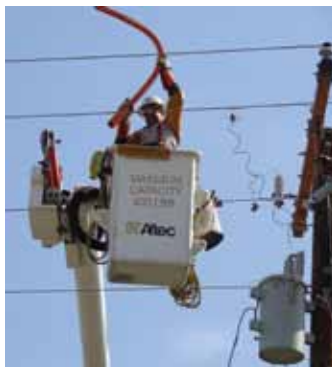
Lineman Roy O'Neal places a line hose over a power line. The line hose helps to prevent lineman from contacting a power line.
