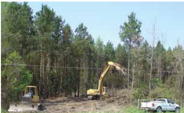
Contractors work to clear a wooded area for the future location of Albemarle EMC's new office building.
