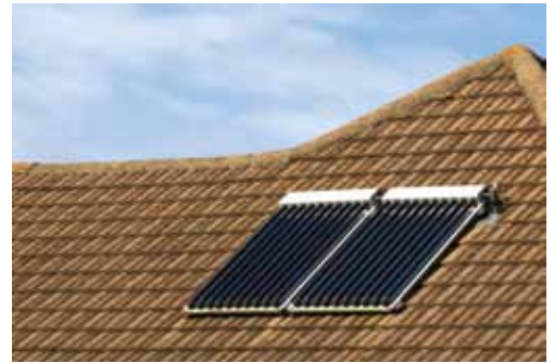
Albemarle EMC offers a $1,000 incentive if you properly install solar water heaters, such as the ones shown.
